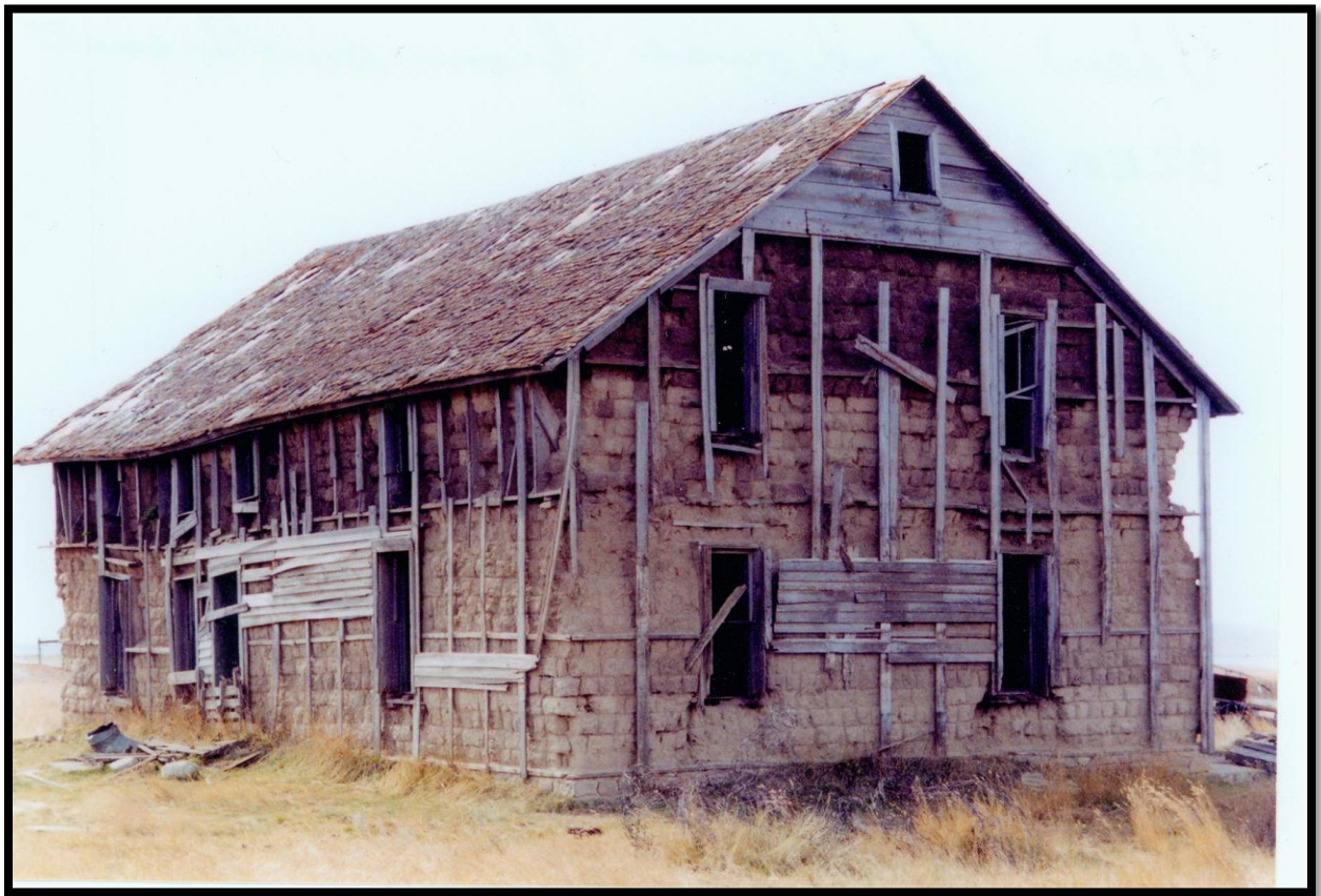
32EM344-George Backhouse home. This is an example of the use of available materials for home construction. Photo Courtesy of Division of Archaeology and Historic Preservation, State Historical Society of North Dakota.
