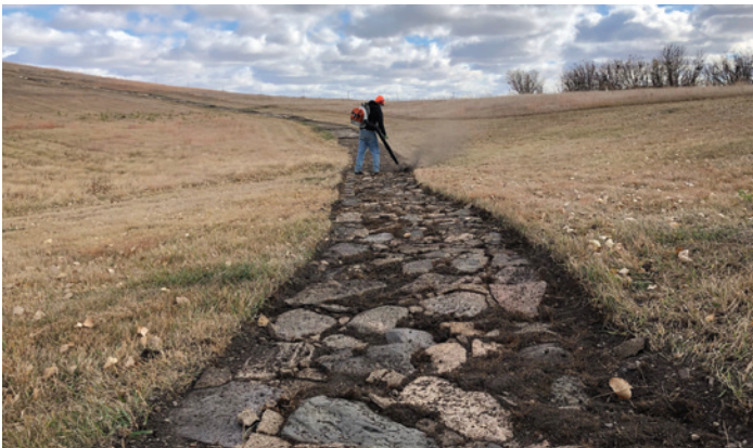
Site Supervisor Stewart Lefevre clears sod off a Works Progress Administration path at Whitestone Hill State Historic Site.
