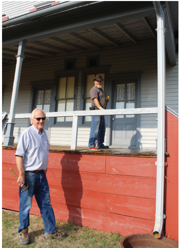
Assistant Site Supervisor Ed Sahlstrom, left, and maintenance staffer Mike Sunday give the porch of the Chateau de Morès a little TLC.
