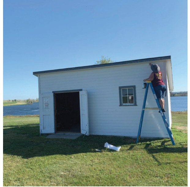
Interpreter Amanda Baumgartner gives the blacksmith shop at Welk Homestead State Historic Site a new coat of paint.
