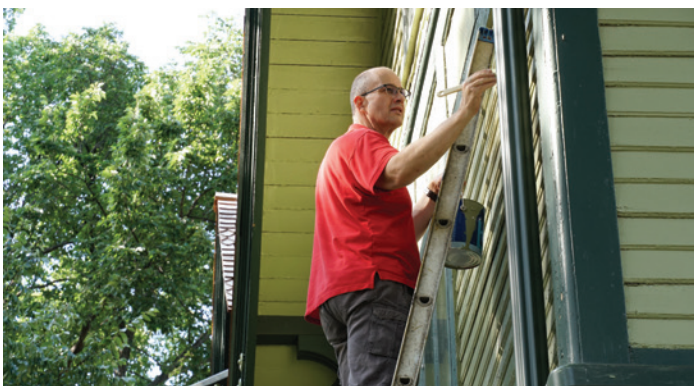
Site Supervisor Johnathan Campbell paints the exterior of the Former Governors' Mansion.
