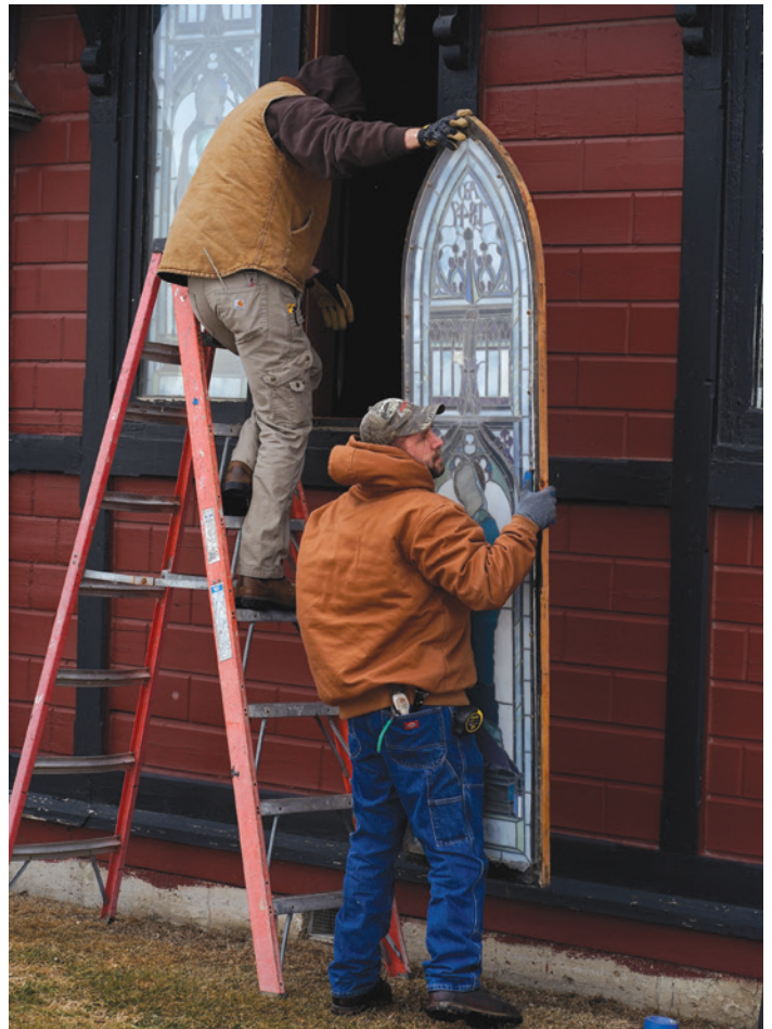
Conservators carefully remove the Leah F. Parkhurst Memorial Windows at Camp Hancock State Historic Site's Bread of Life Church for restoration. The windows were made in 1882 by prominent stained-glass designer John La Farge.
